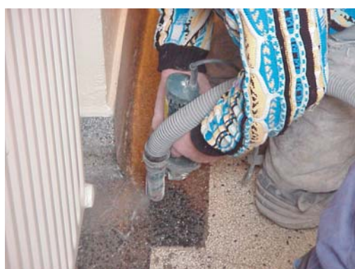
Incorrectly placed local exhaust ventilation affects effectiveness
