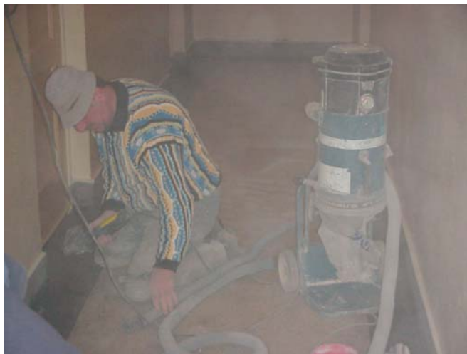
Sliding connections can disconnect easily
